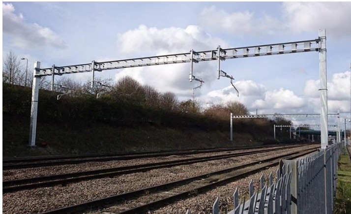
Figure 15: Electrification infrastructure near Didcot Parkway
